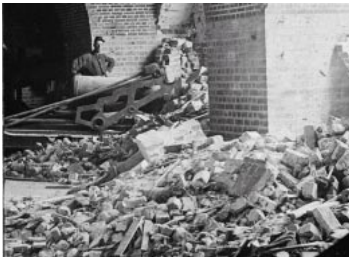
Casemate damage in the interior of Fort Pulaski after the bombardment. Brick could not withstand rifled cannon.
